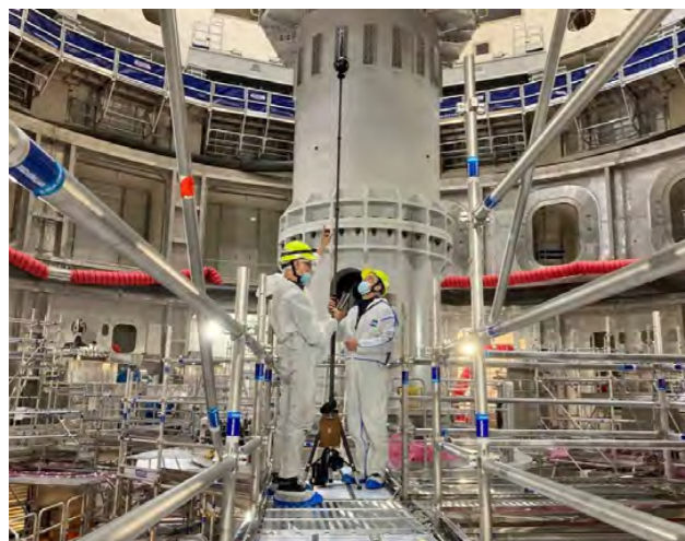
Two workers stand in the central Tokamak pit, a 30-metre-tall x 30-metre-wide space where the assembly of the ITER machine is proceeding from bottom up. April 2022. ©ITER Organization
