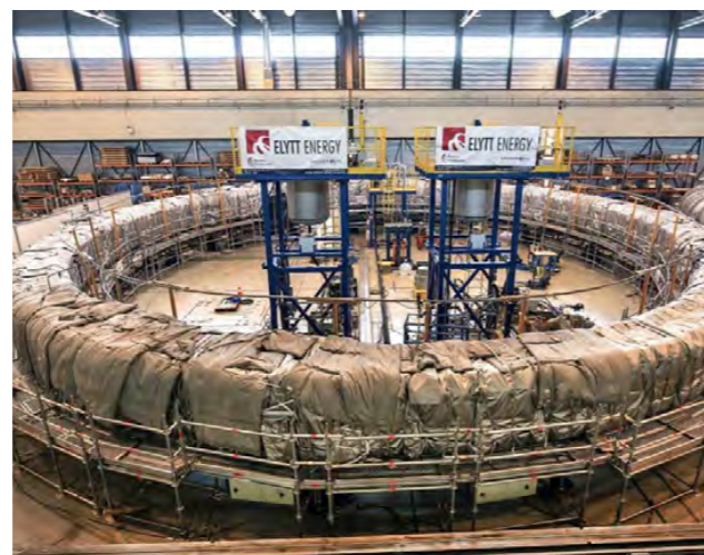
In July, contractors to the European Domestic Agency carry out the vacuum pressure impregnation (VPI) of poloidal field coil #4. July 2022. ©ITER Organization
