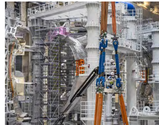
Against the backdrop of vacuum vessel sector assembly, China Nuclear Power Engineering (CNPE) consortium members are preparing to move a 100-tonne central solenoid module. February 2022. ©ITER Organization
