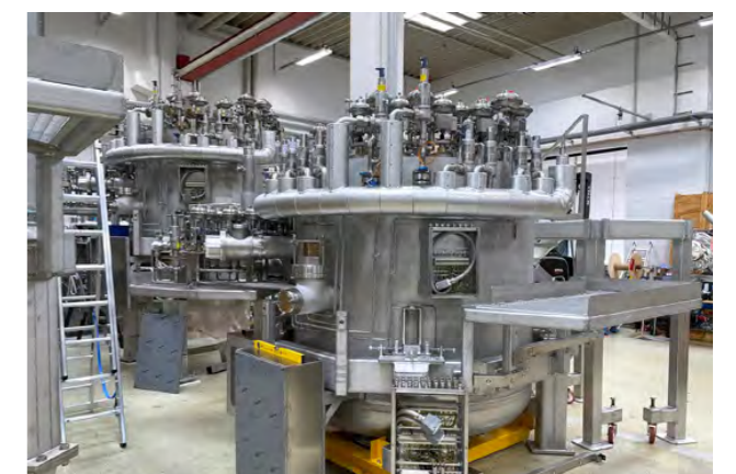
Two cold valve boxes (CVBs) in the workshop of Research Instruments, Germany. F4E, in collaboration with Research Instruments (RI) and Cryoworld, has already completed four CVBs. August 2022. ©RI
