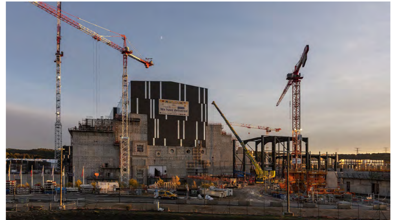
Against the concrete structure of the Tokamak Complex, the frame of a new building is emerging: the tall High Voltage Building that will house the high voltage equipment for neutral beam injection. November 2022. ©ITER Organization
