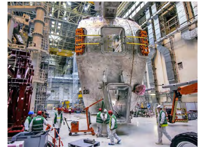
On 12 September, vacuum vessel sector #8, from Korea, was transferred from the upending tool (left) to the available sector sub-assembly tool on the other side of the Assembly Hall. September 2022. ©ITER Organization
