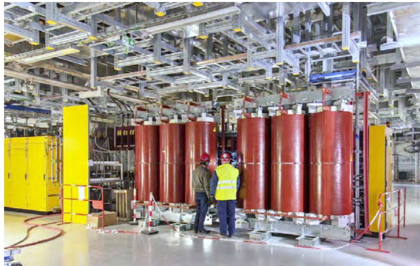
One of the two sets of high-voltage power supplies for the electron cyclotron resonance heating (ECRH) system installed on the second floor of the Radio Frequency Building. November 2022. ©ITER Organization.
