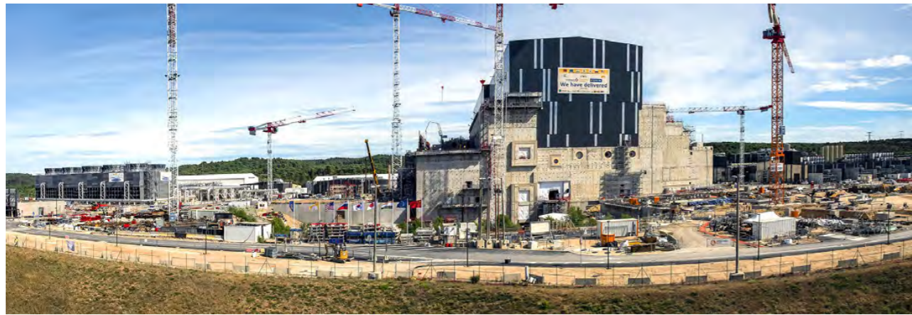
At 25 metres tall, the High Voltage Supply Building, will partially obscure the Tokamak Complex, rising several metres higher than the four transmission line openings that are visible in the concrete facade. July 2022. © ITER Organization
