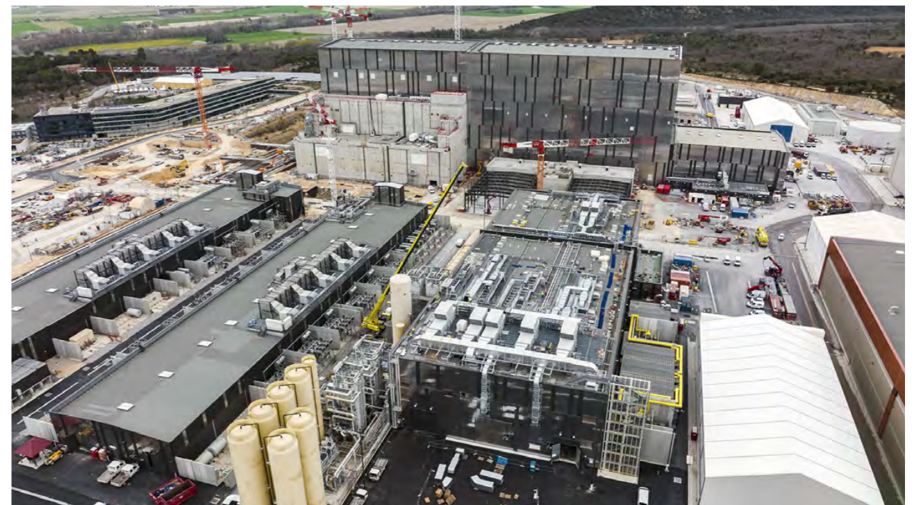
Aerial view of ITER construction site, where steel frame works of the Fast Discharge facility can be seen on the right of the Tokamak Complex, Cadarache, France, April 2022 © ITER Organization
