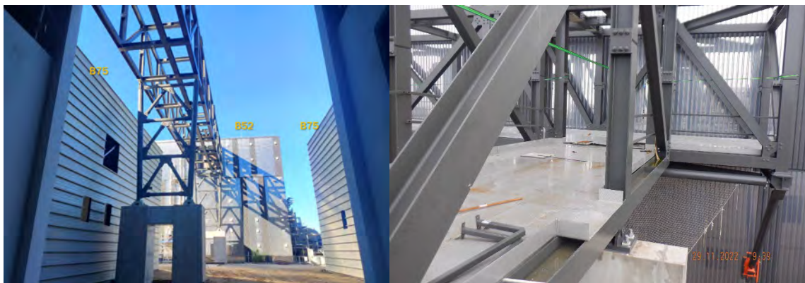
Figure 5: TB12 (Demathieu Bard) Cryoline bridge (connecting Cryoplant Building B52 with Tokamak Building B11) metallic structure installation (left) and flooring and roofing installation (right).
