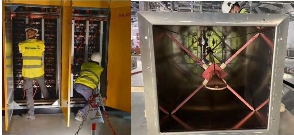
Figure 36: (left) Connection of the power converter modules for the charging procedure carried out during the installation of the 2 first Power Supply sets in the ITER RF Building, Cadarache, France, May 2022.; (right) Installation of the coaxial Feeder Line that
