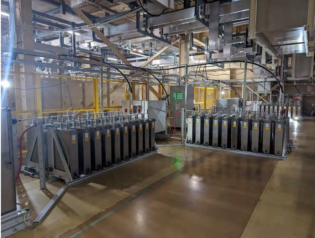
Figure 39: JT-60SA Booster Power Supply Filter
