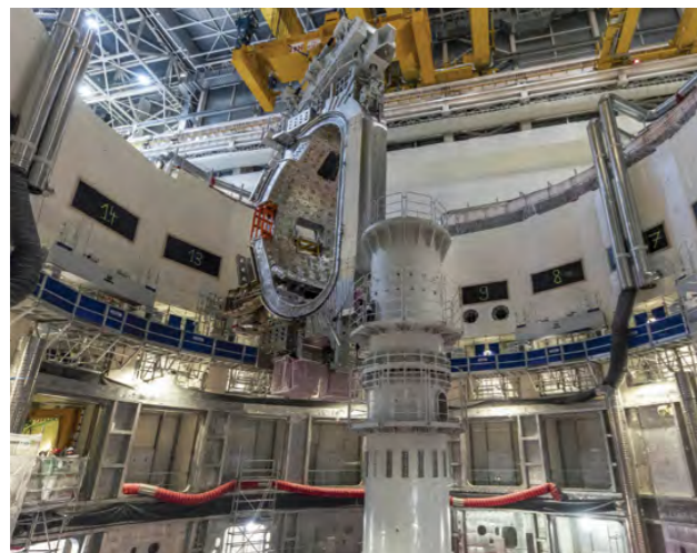
Sector module #6 lifted from the assembly pit and transported to the sub-assembly tool to remove components and perform maintenance. July 2023. ©ITER Organization
