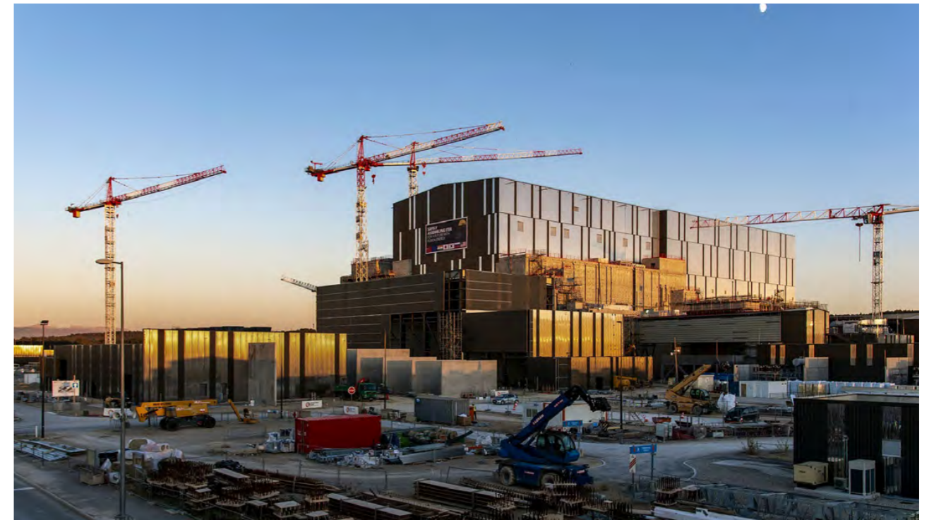
The banner on the façade changed to a message of commitment: "Safely assembling ITER." November 2023. ©ITER Organization
