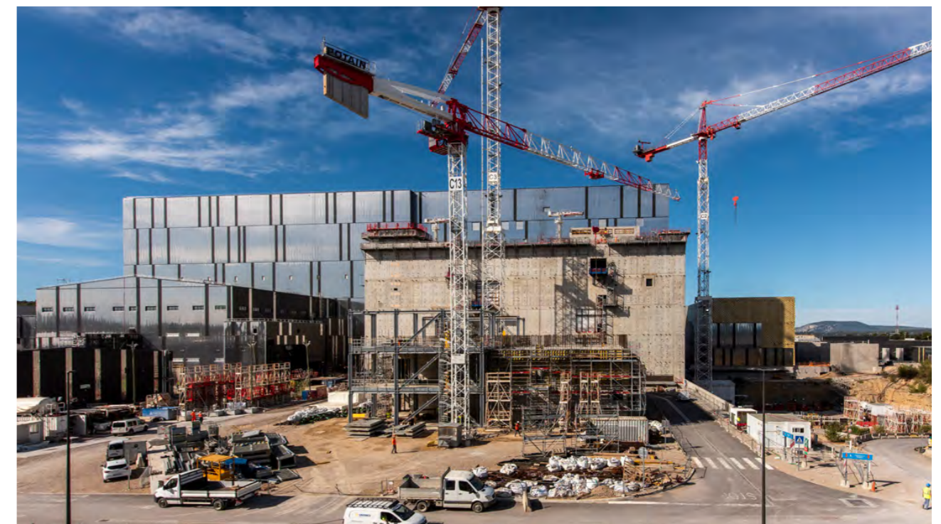
Civil works on the Tritium Building are over and tall cranes will be dismantled, as the building is completely framed out. December 2023. ©ITER Organization
