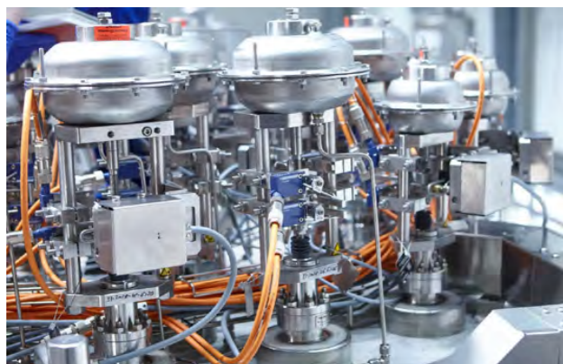
Close up of the valves in the Cold Valve Boxes, that ITER will rely on in order to attain the vacuum conditions in its vessel. 2023. ©RI
