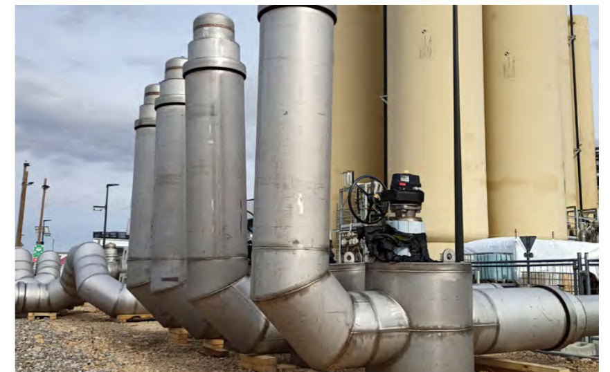
The quench line headers stand in the cryoplant storage area. October 2023. ©F4E
