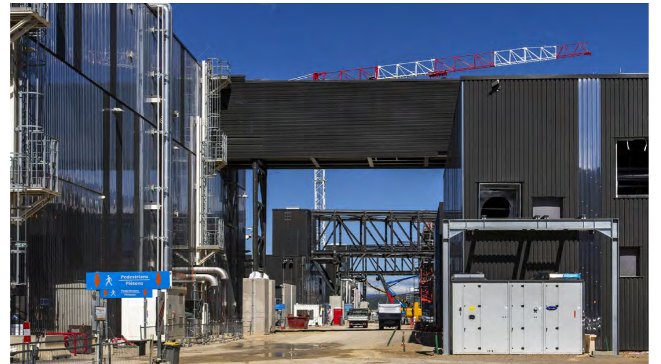
Three new bridges to the Tokamak Complex: the cryoline bridge (foreground) will channel cryogenic fluids, and the two busbar bridges will allow transport of electrical busbars from the Magnet Power Conversion. August 2023. ©ITER Organization
