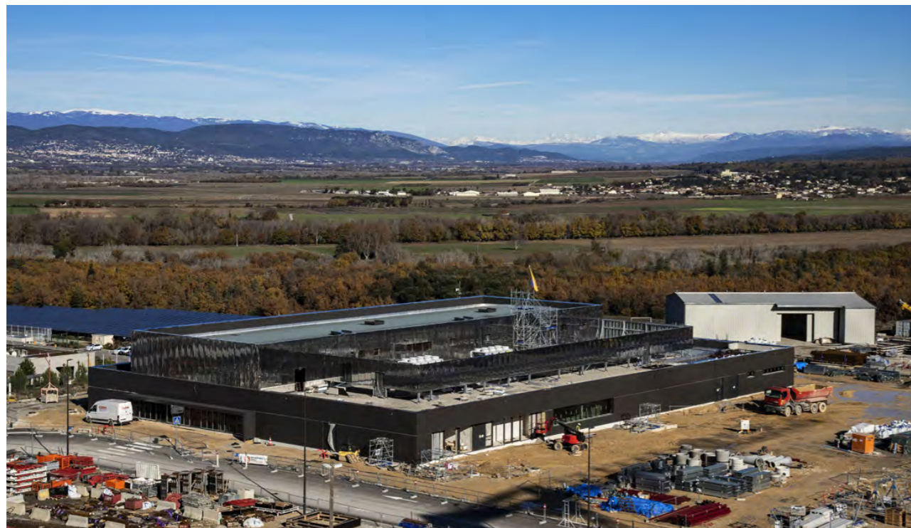
Steady progress in the Control Building, connected underground with the ITER Organization Headquarters. 2023. ©ITER Organisation
