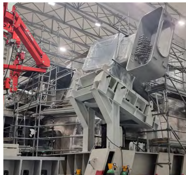
Installation of in-wall shield blocks (poloidal segment 2- poloidal segment 3 joints) of Europe's vacuum vessel sector 5 in the factory of Westinghouse Mangiarotti, Italy, 2023. ©F4E
