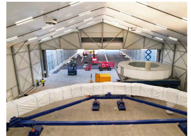
PF4 and the smaller PF6 in storage on the ITER site. September 2023. ©ITER Organization
