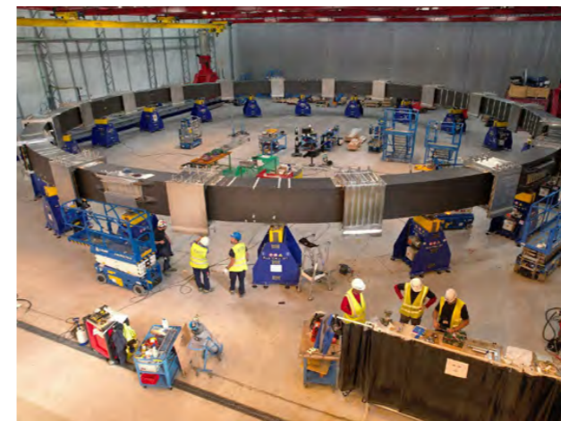
PF3 assembled before the cold test. After its delivery, the whole facility will be handed over to ITER Organization for other assembly purposes. September 2023. ©ITER Organization
