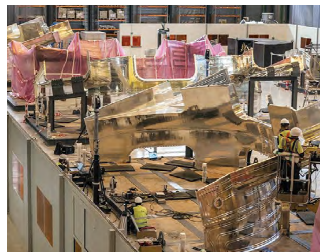
Outboard segments of thermal shield await disassembly by contractor teams at the Poloidal Field coils factory on site. August 2023. ©ITER Organization
