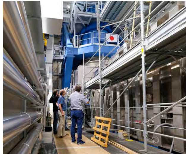
Inside of the MITICA bunker with the vacuum vessel on the right and the last part of the 1MV transmission line in blue. September 2023. ©ITER Organization
