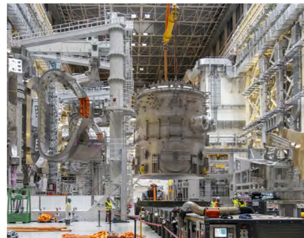
Procured by India, designed and manufactured by Linde Kryotechnik AG in Switzerland, three of the five auxiliary cold boxes—part of the cryogenic distribution system—have been pre-positioned in the Tokamak Building. December 2023. ©ITER Organization
