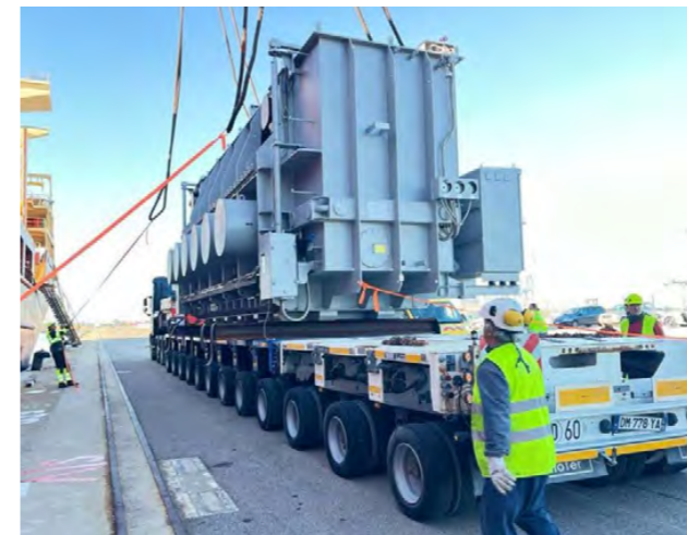
The last of Korea's 18 AC/DC transformer/converter units made it to ITER, where it will be integrated in the power supply system. December 2023. ©ITER Organization
