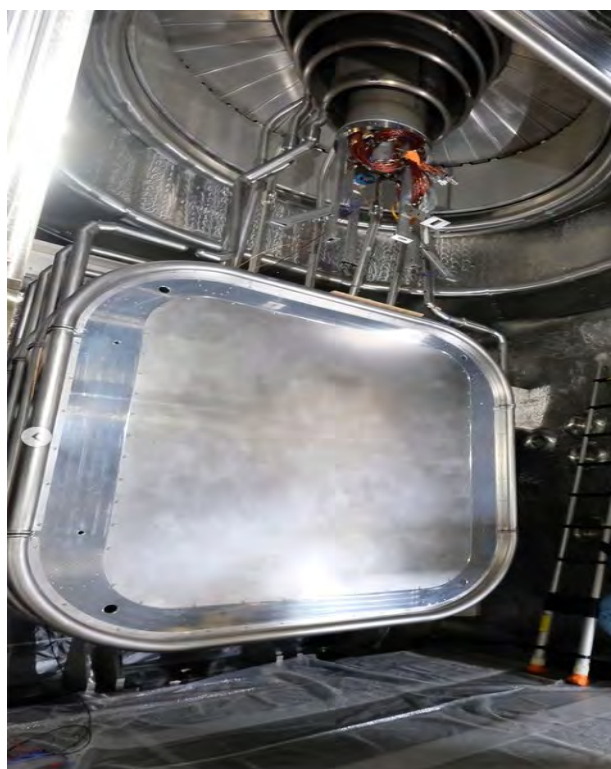
Figure 29: Beam Source mockup installed at MITICA for HV Holding Tests
