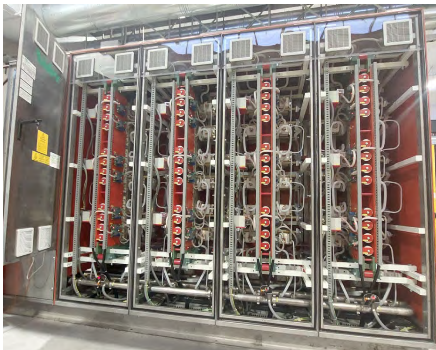
Figure 31: Rectifier unit of the Acceleration Grid Power Supply system of ITER, during Factory Acceptance Testing.
