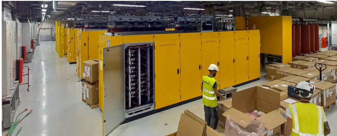
Figure 38: The eight EU High Voltage Power Supplies are installed in the ITER building #15, ready for commissioning.
