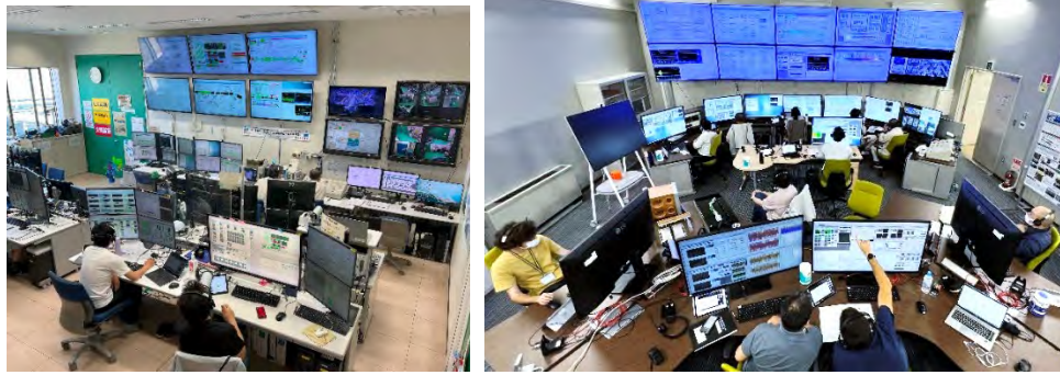
Figure 45: IFMIF/LIPAc control rooms on Rokkasho site: Left local control room, right central control room.
