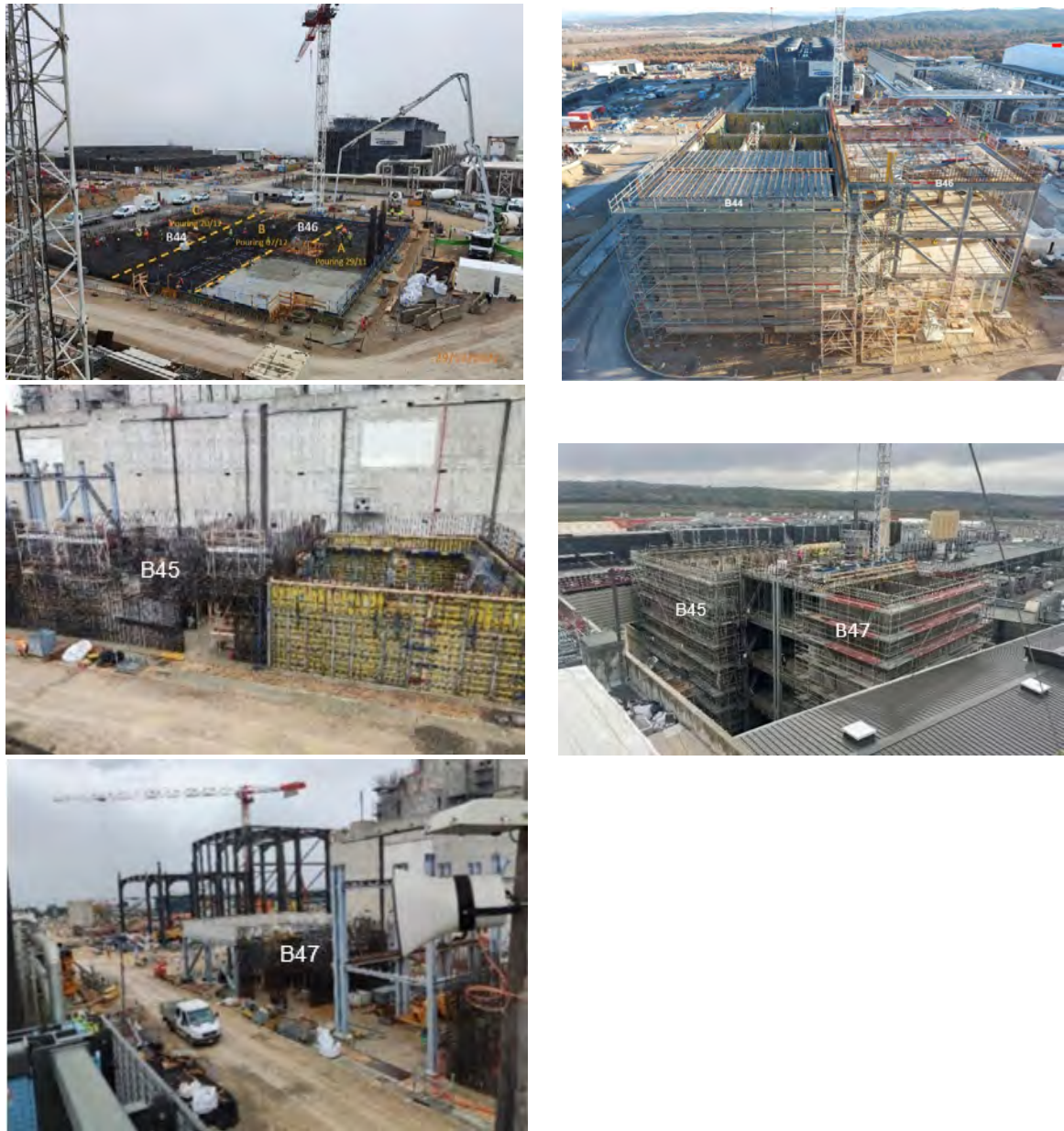
Figure 3: TB13 (Ansaldo - Monsud) B44, B45, B46 and B47 Power Supply and Distribution Buildings work status in November 2022 (left) versus December 2023 (right) Photos: ©F4E
