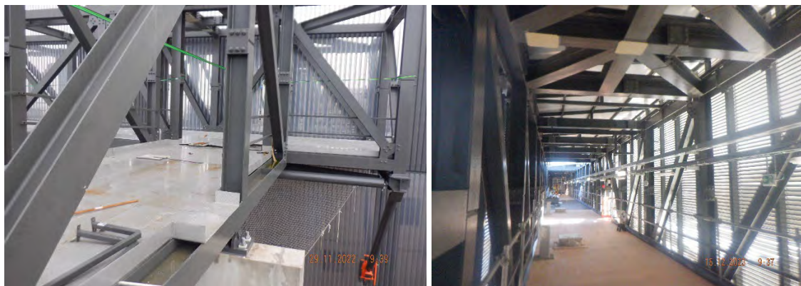
Figure 5: TB12 (Demathieu Bard) Cryoline bridge (connecting Cryoplant Building B52 with Tokamak Building B11) (left) in November 2022 versus December 2023.
