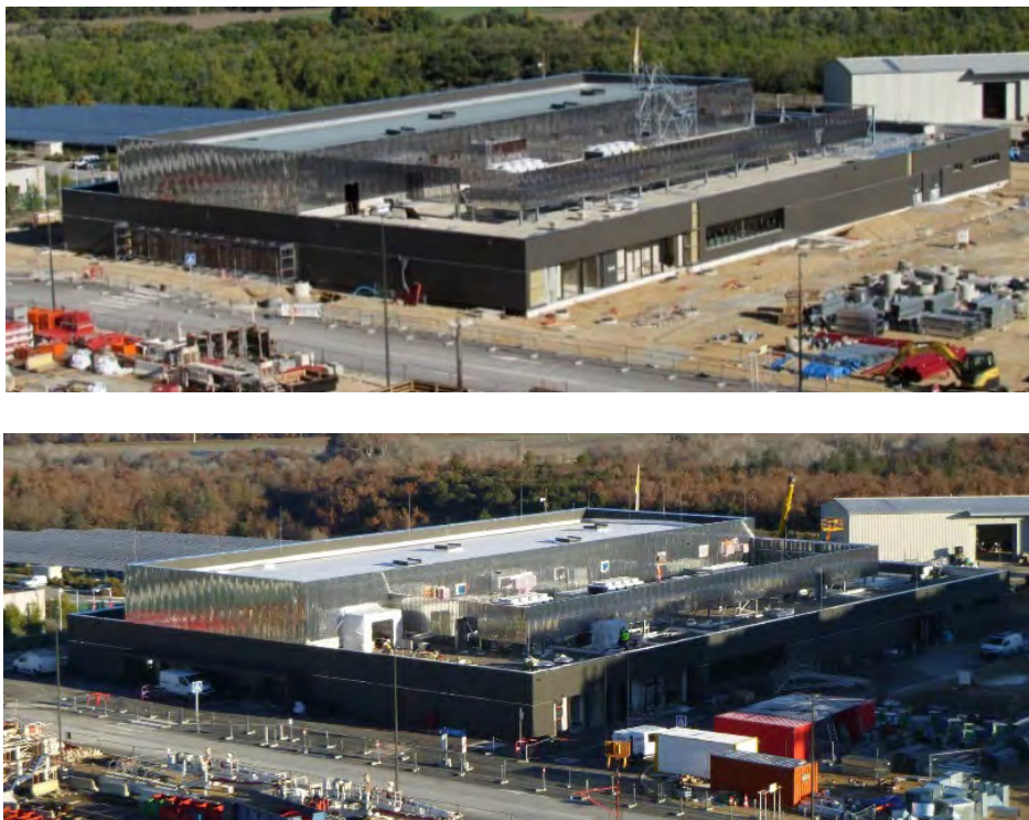
Figure 4: TB12 (Demathieu Bard) B71 Control Building North work status in November 2022 versus December 2023
