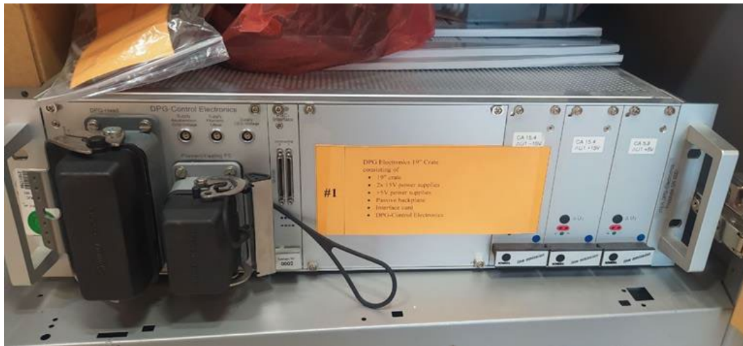
Figure 55: Chassis containing the electronics that connect the pressure gauge to its power supplies and to the system that reads and records its data
