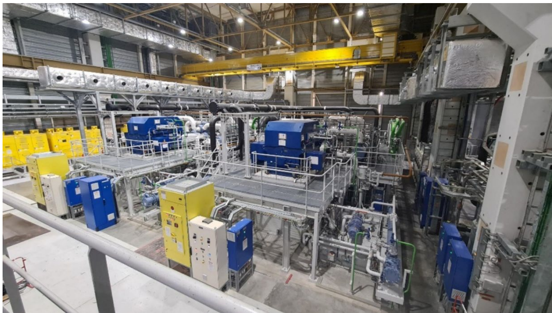
Figure 35: LN2 Plant compressors operational on site
