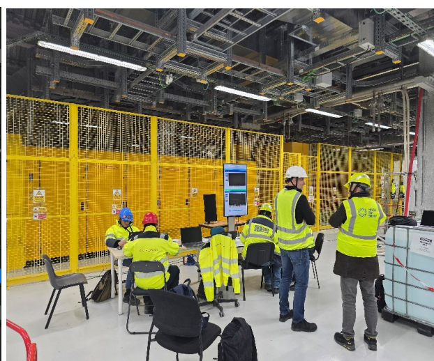
Figure 43: EC Power Supplies Unit 05 Site Acceptance Test (SAT)
