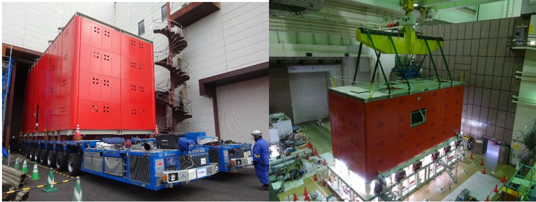
Figure 78: The moving (left) and installation of the large high voltage table for the negative NBI sources
