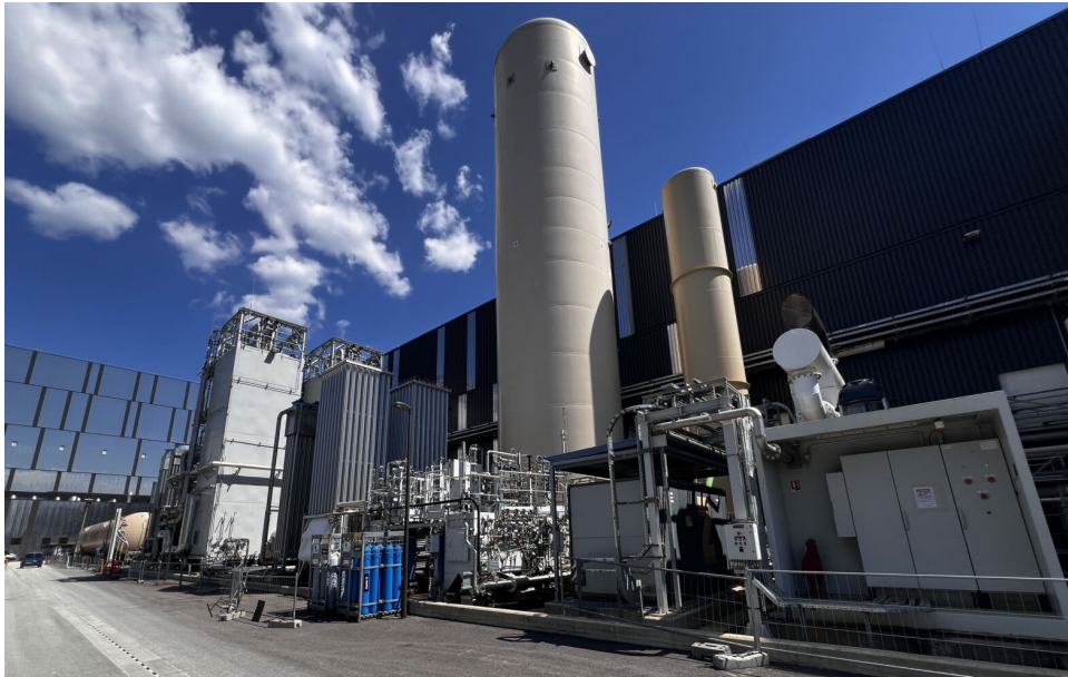
Figure 34: Exterior view of the ITER cryoplant, with the liquid nitrogen tank towering over the large facility. April 2025. ©F4E
